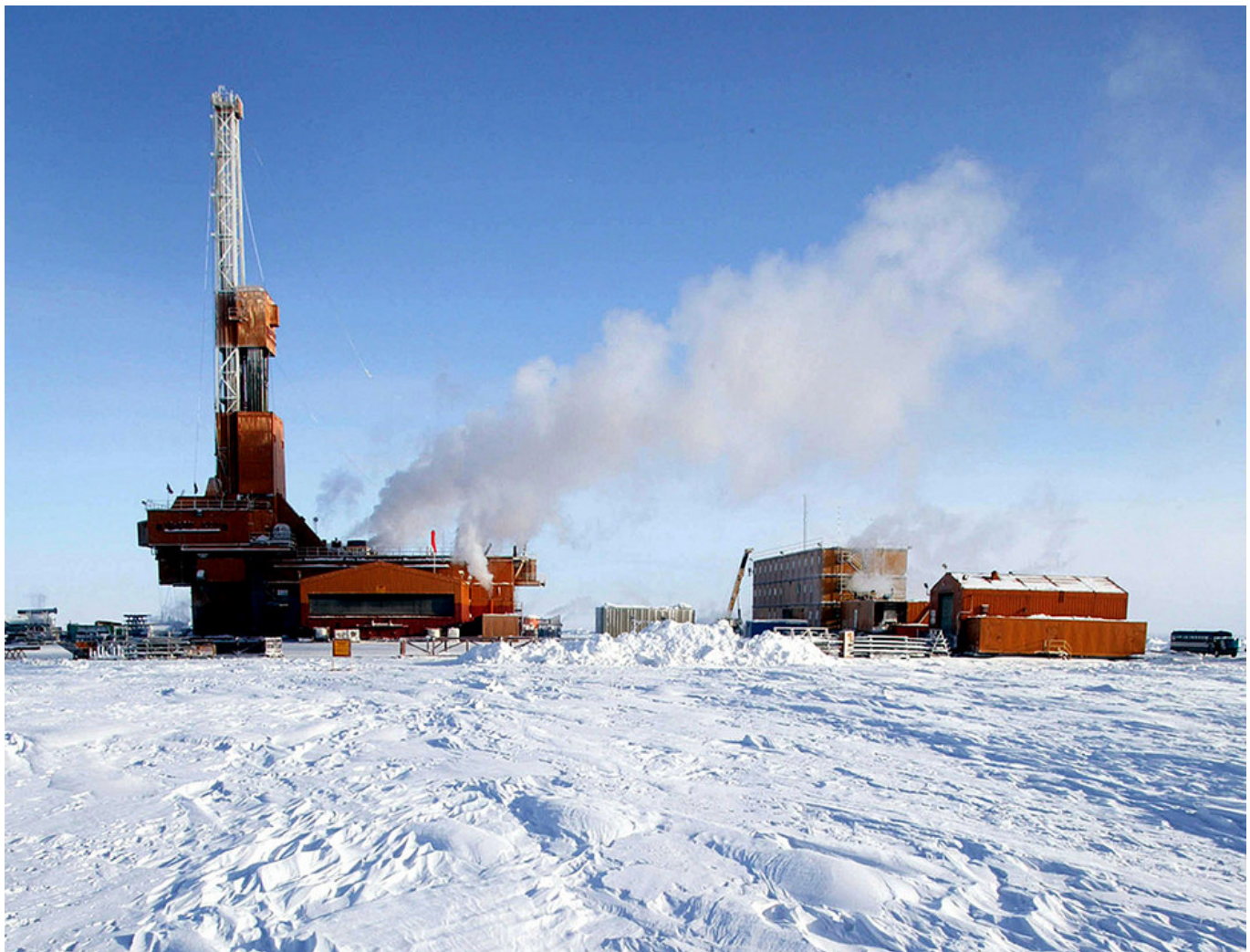
Drilling operations at the Doyon Rig 19 at the ConocoPhillips location in the National Petroleum Reserve-Alaska. | Judy Patrick/AP Photo
